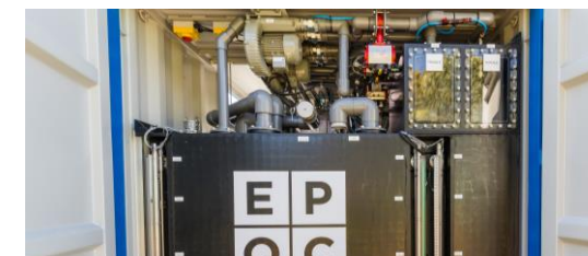
Final (tertiary) Concentrate Tank
